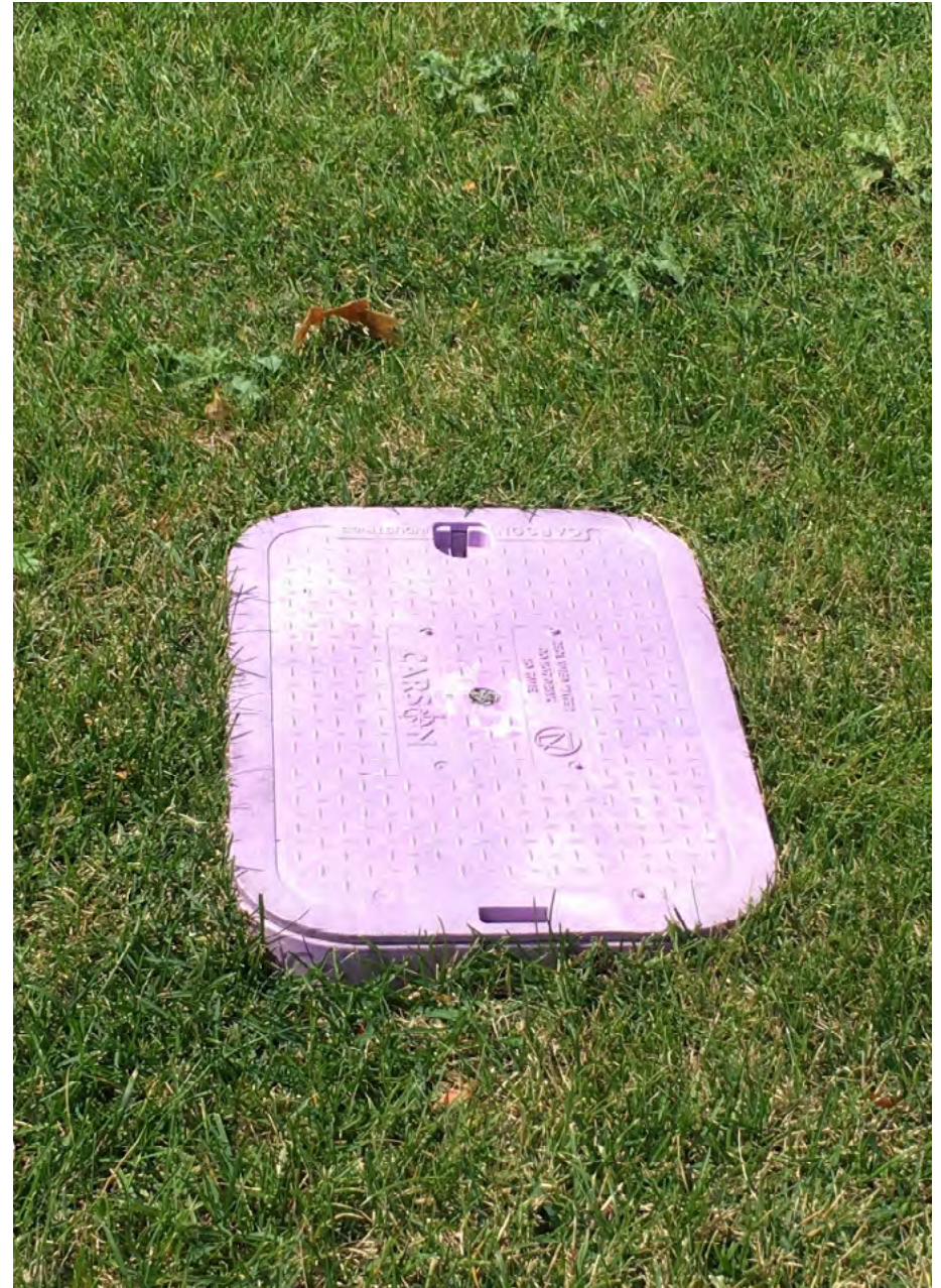
Figure 7. Reclaimed water system in Westminster, Colorado
